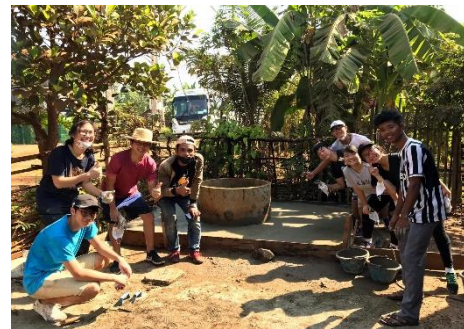
Well paving at a local village
